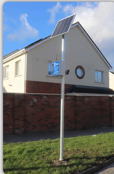
Overheight Vehicle Detection Station
