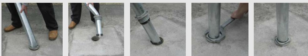
Removing damaged post. Damaged post removed. Install new post. Lock new post in position. New post installed.
